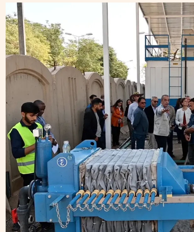
UNICEF and the United Nations Assistance Mission for Iraq (UNAMI) collaborated to install an MBBR wastewater treatment system at the UNAMI office building. MBBR systems installed across Iraq help reduce water shortages worsened by climate change. ©UNICEF Iraq
